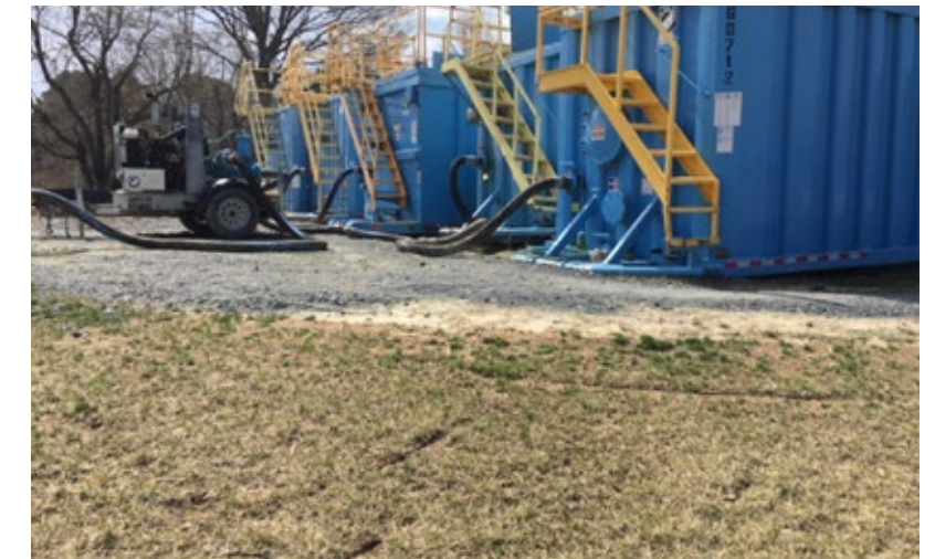
'Rain for Rent' storm water filtration system at K. Hovnanian's® Four Seasons at Kent Island community
